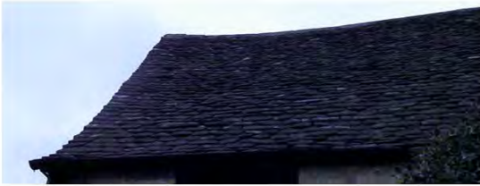
Whoosh at the base of a stone slated roof
