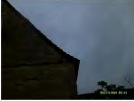
whoosh at the base of a stone slated roof
