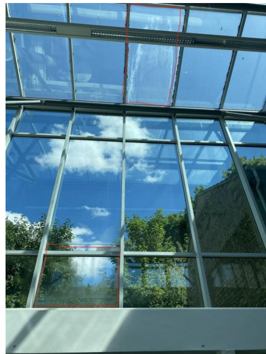
Photograph (iv) failed panels marked red
