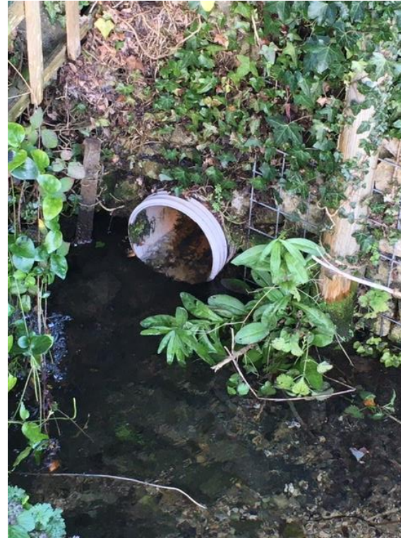
Figure 4 Drainage outlet at Court Brook 15th January 2020 (after storm Brendan)
