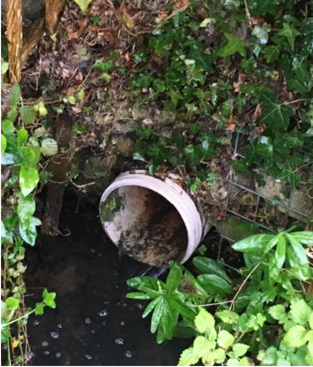
Figure 1 Drainage outlet at Court Brook 12th December 2019 (wettest December on record)
