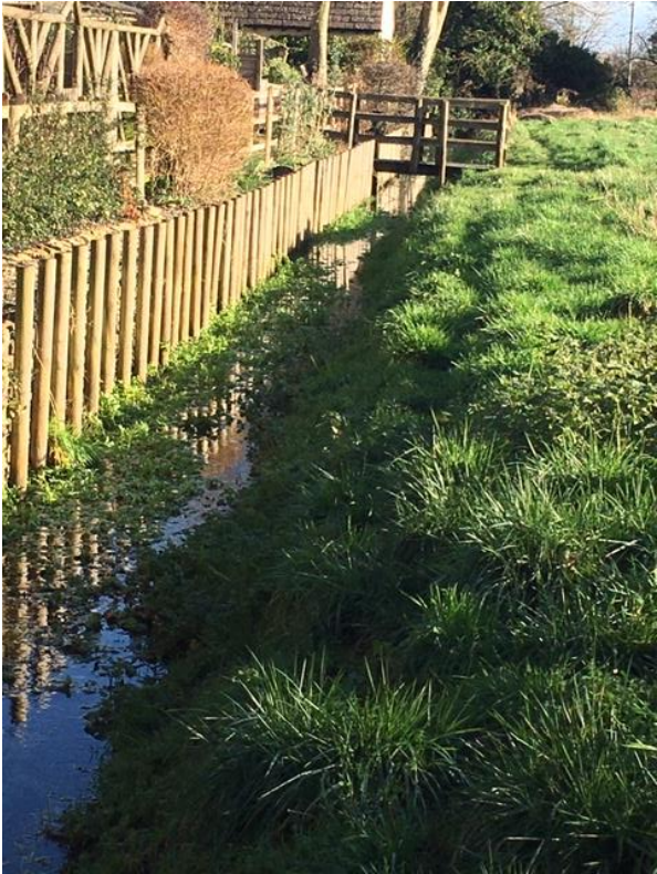
Figure 5 Drainage ditch 15th January 2020 (after storm Brendan)
