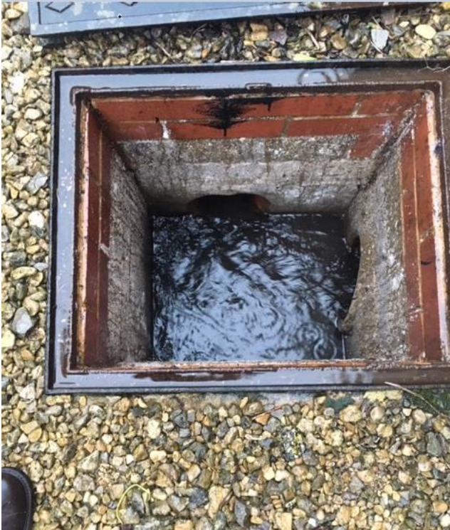
Figure 3 Manhole inspection point 12th December 2019 (wettest December on record)
